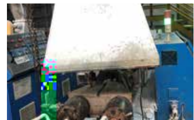
Exhaust gas treatment device in a workshop
