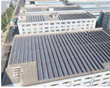
Solar PV Panels on the Roofs of Plants
